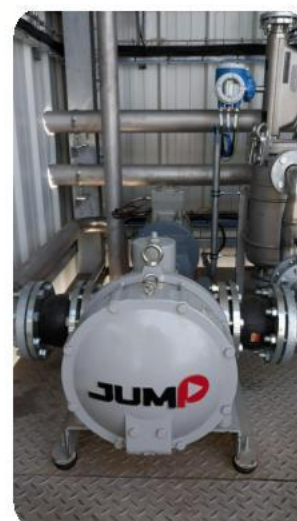
Pumping unit JE24s
